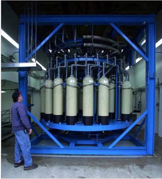
Steve Quirino, a Suffolk County Water Authority field operator, checking the filtering tanks in Northport. Experts wonder how much water Long Island has left.
